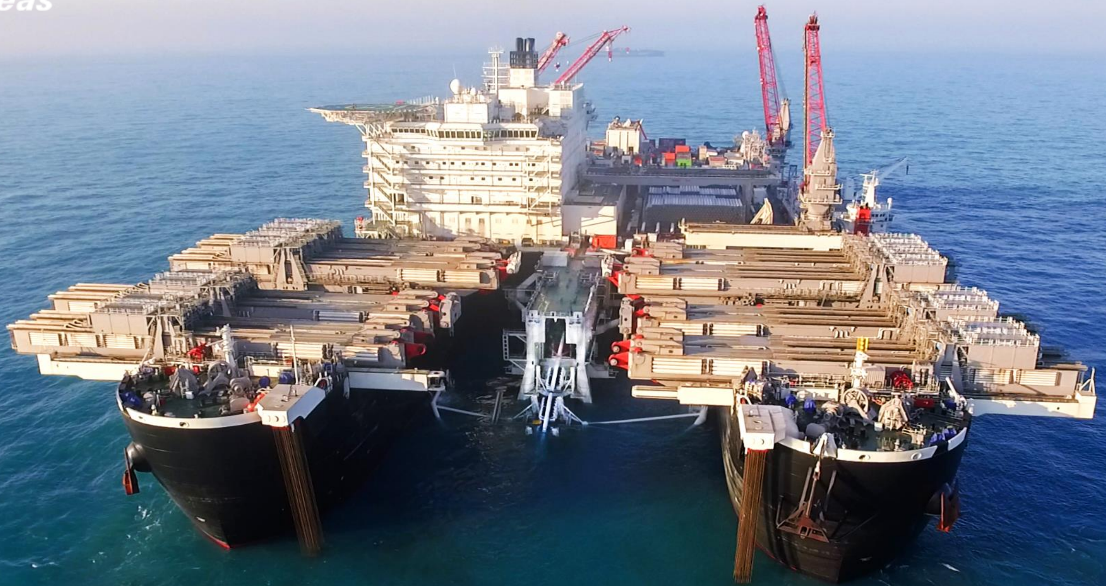
Pioneering Spirit installing the TurkStream gas pipeline in the Black Sea, July 2017 5
