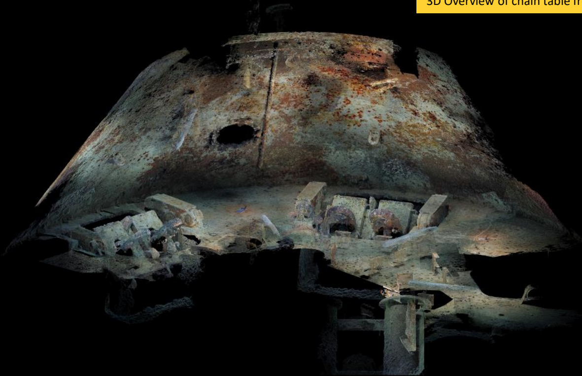
3D Overview of chain table from within FPSO turret
