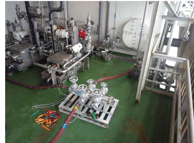
Typical steam equipment: small footprint
