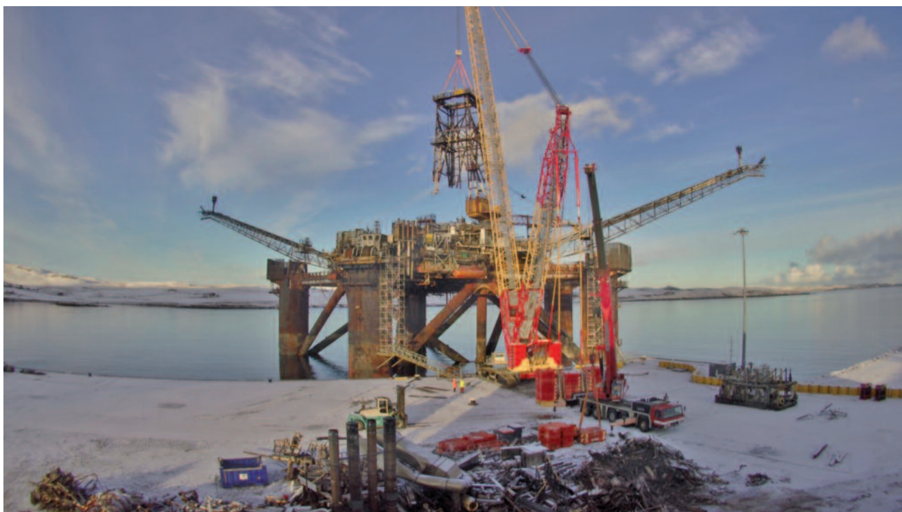
Figure 6: Decommissioning of the Buchan Alpha at .Dales Voe by Veolia. Source: Veolia.
